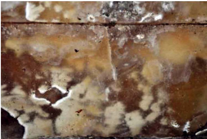
Abb. 6: Villa A (Oplontis), Room 14 alabaster threshold
